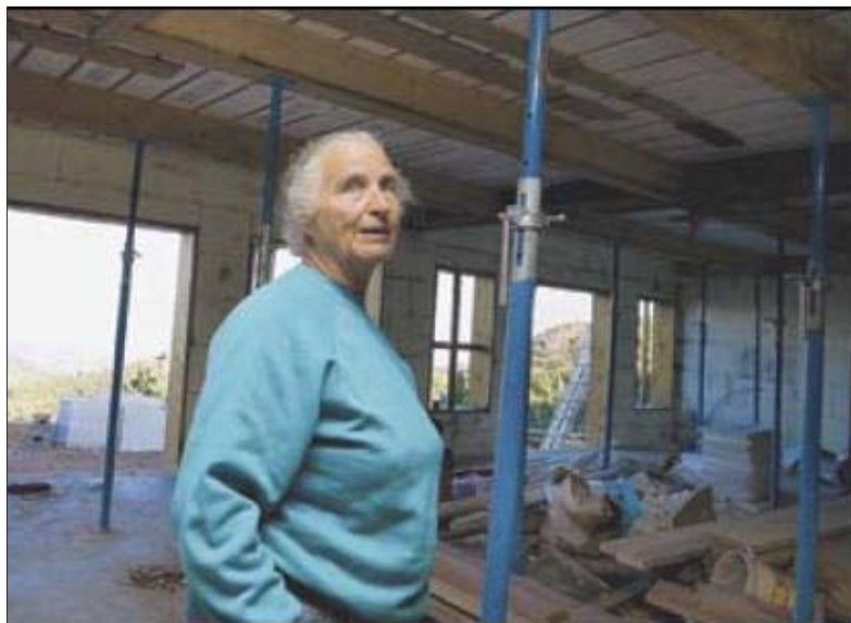
Natasha Kent stood in what will be the basement of the home she's building. her husband, james Olsen, has stayed on the sidelines in recent months because he broke his leg in june.
